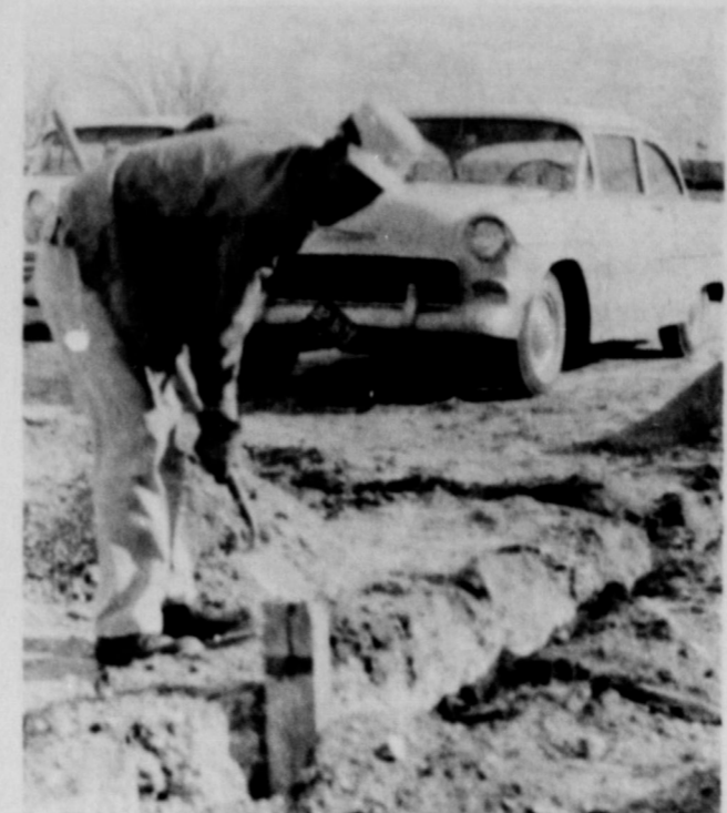
BELIEVE IT OR NOT , An electrician not a ditch digger. However, it just goes to prove the Versatility of a business man who tries real hard to please a customer in this fast moving world of today. Actually, Carlis Bills was discovered during these electric lines at the A to Z Fertilizer Plant. (Actually he's not to fond of diggin ditches)
