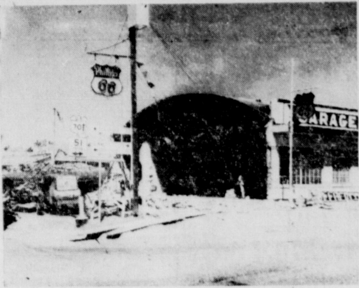
REMODELING — Pictured is the Springlake Motor Supply in Springlake which is now undergoing a "face-lifting". The Phillips 66 Service Station and garage, owned and operated by Elroy Wisian, is being moved back several feet from the recently completed four-lane highway through the town. When finished, the building will feature a brick-veneer front with several large plate glass windows and separate wash and grease rooms.
