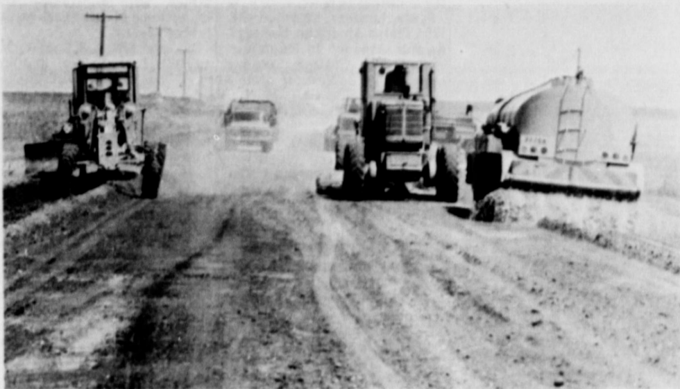
TO ELIMINATE THE Springlake School road from being closed, due to high water, as it was several times last year, the State highway department began operations last week to raise the road approximately three feet, in order to prevent the water from overflowing the road.
