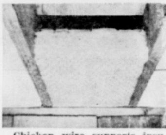
Chicken wire supports insulating batt of mineral wool between joists of crawl space floor.
