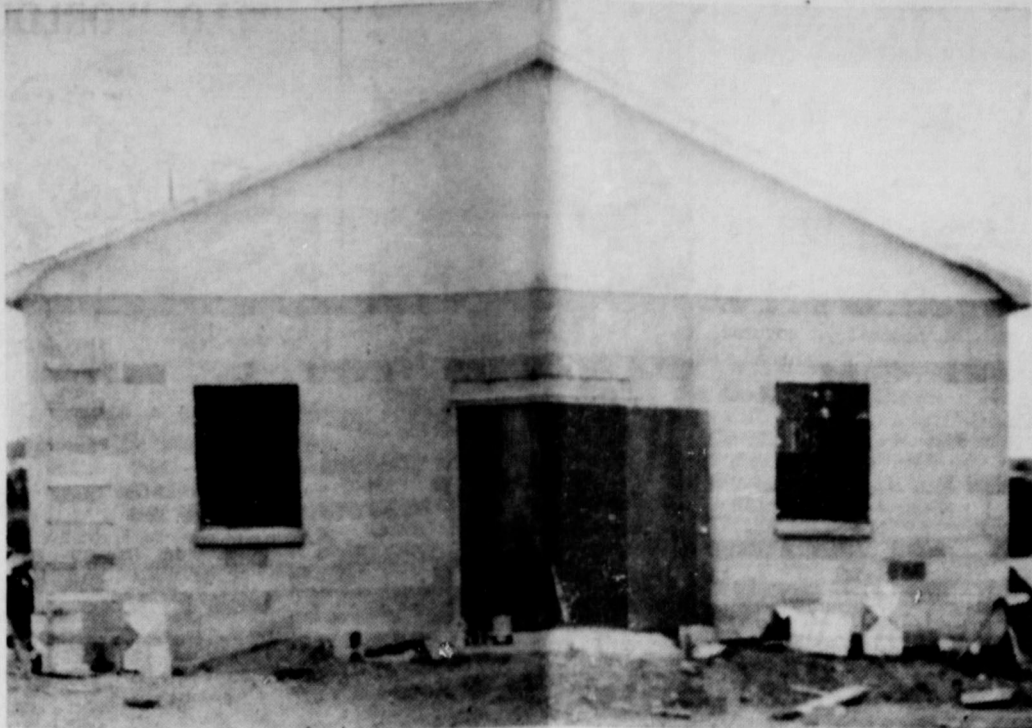
NEGRO BAPTIST CHURCH — This 30'x50' building is completed. Services are held each morning and evening. The building is constructed of cement blocks and has seating capacity of approximately 150 persons.
