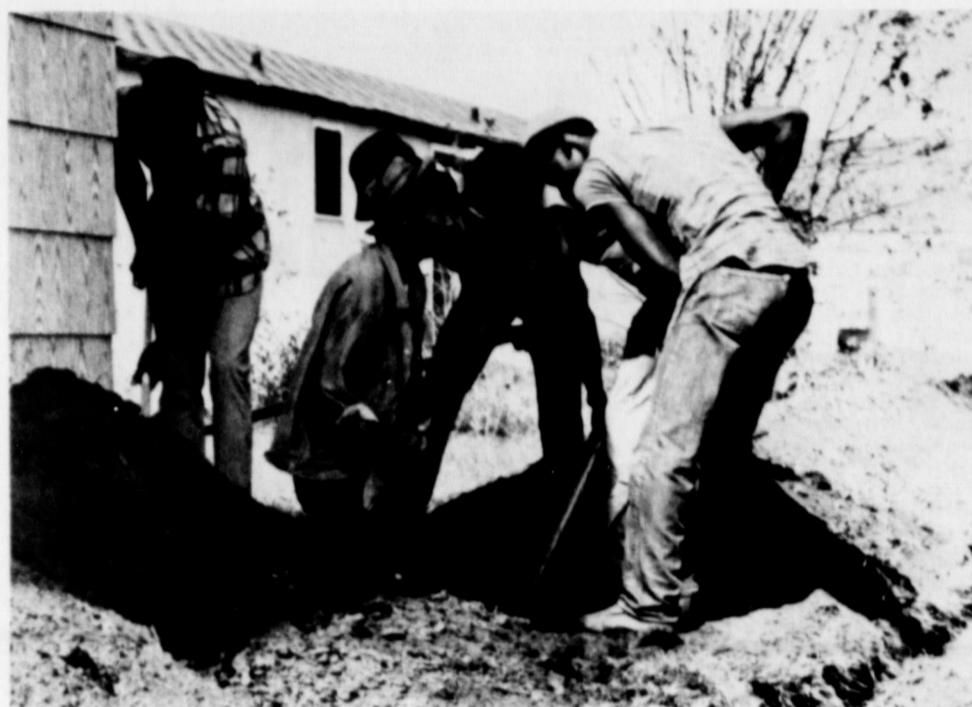
A LARGER SEWER LINE goes in on the faculty row of the Springlake-Earth campus. Increased housing on the campus has made the improvement necessary.
