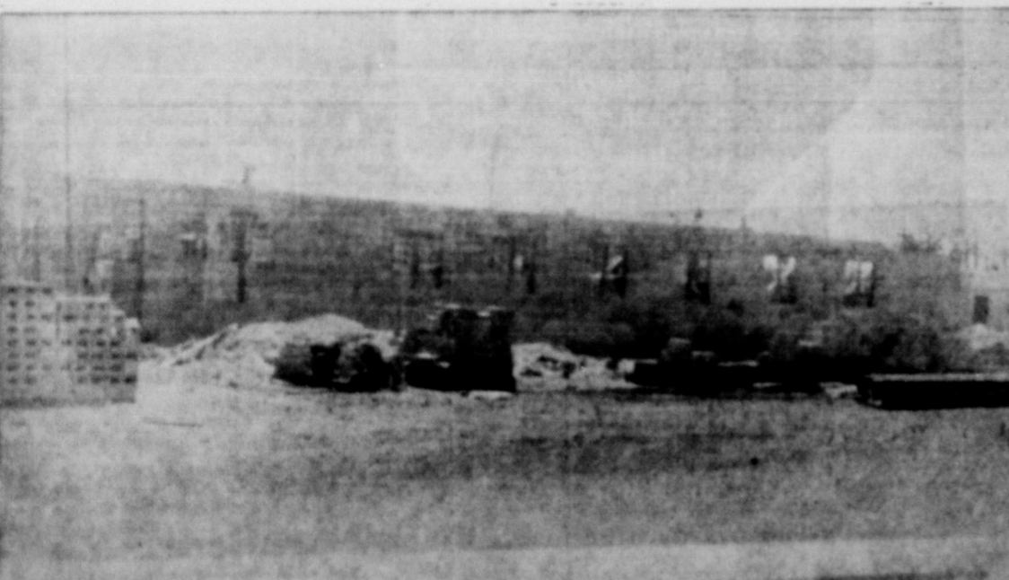
UNDER CONSTRUCTION is this new 15 room Clinic Hospital being built by Dr. F. B. Faust. Dr. Faust came to Earth in June 1955. The new hospital adds to the enormous growth Earth has had the past two years.
