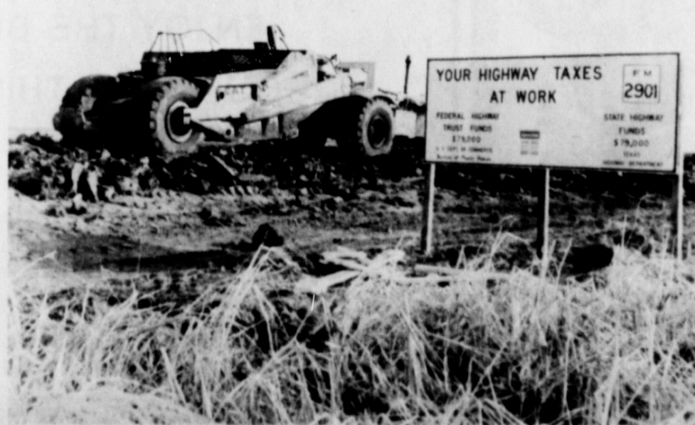
WORK HAS BEGUN ON RAISING FM 1055 north of Earth approximately 2 to 3 feet where water has been getting over the highway. Preparations are also being made to begin to work on the road that runs east and west by Springlake-Earth School between FM 1055, and Highway 385.
