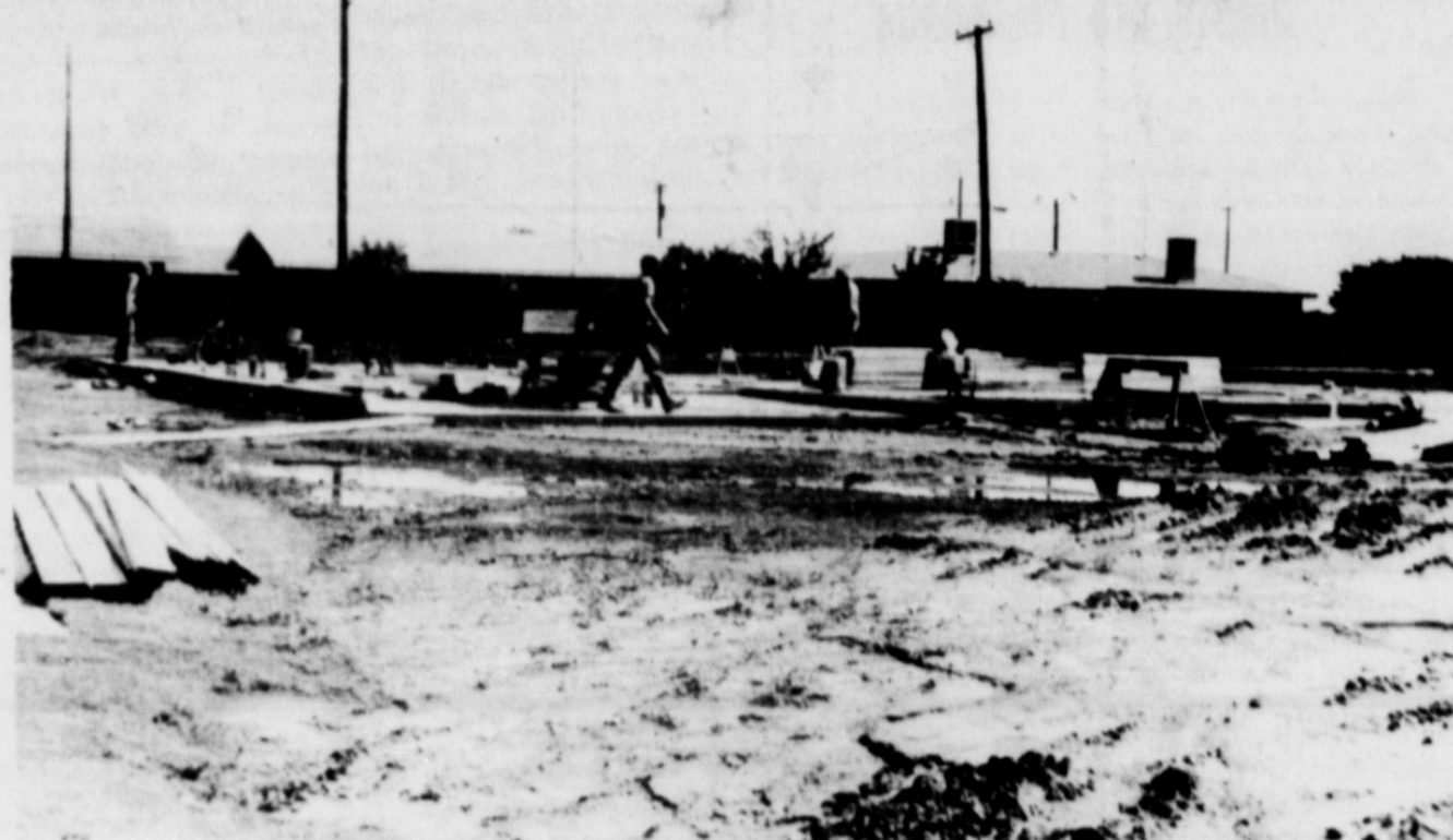
NEW HOME UNDER CONSTRUCTION... This new home now under construction in Hite Park Addition is the home of Mr. and Mrs. W. O. Jones.
