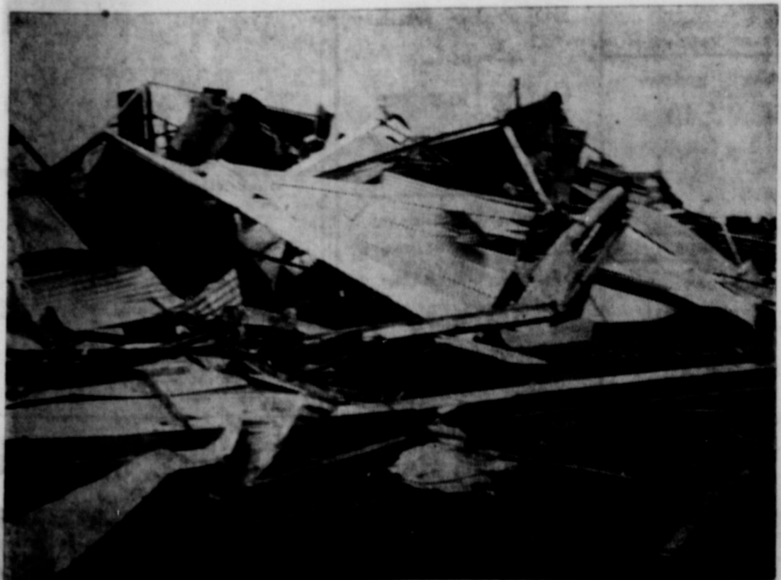
TOTALLY DESTROYED — Is the Lumsden-Perkins Gin located four miles west of Littlefield in which several persons were trapped temporarily in the debris of the gin, behind which they had driven their cars for protection.
