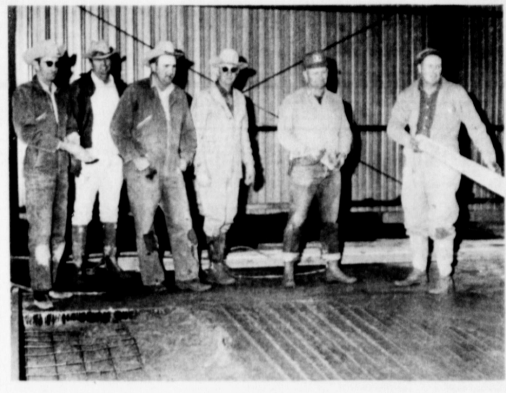
THIS HELPFUL SEXTET shown above are among those of the Springlake-Earth Community donating time, money, and effort to complete the concrete floor for the FFA Livestock barn. Left to right, L. D. Henderson, Thurman Lewis, Bud Matlock, Joel Jones, J. W. Deer, and Tommy Alair.
