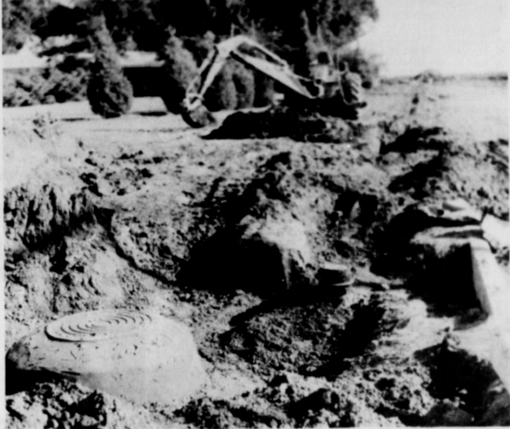
THE WATER AND SEWER EXTENSION PROGRAM nears completion in the Hite Park Addition, as workmen prepare to cover up the ditches as shown in the picture. The additional water and sewer extension was needed in the addition to accommodate Highlight Homes housing project that is expanding at a rapid pace.
