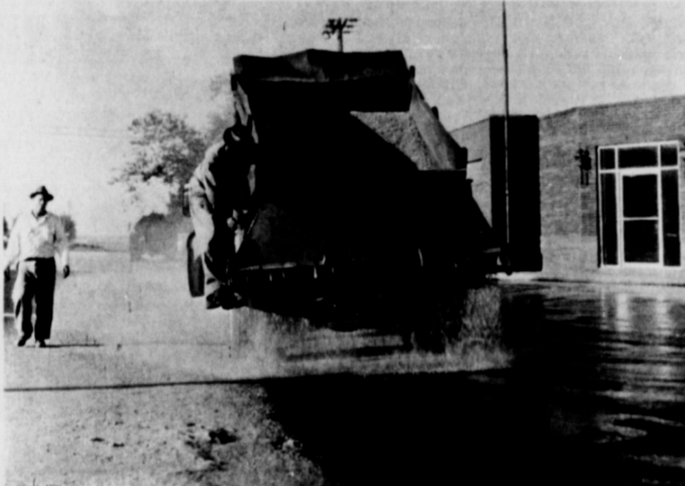
STREET REPAIR IN PROGRESS... All Streets in the city are taking on a new look as all the paved streets are being patched and repaired in the city. The paving repair is being done by Mc Nally Construction Company, Lubbock.
