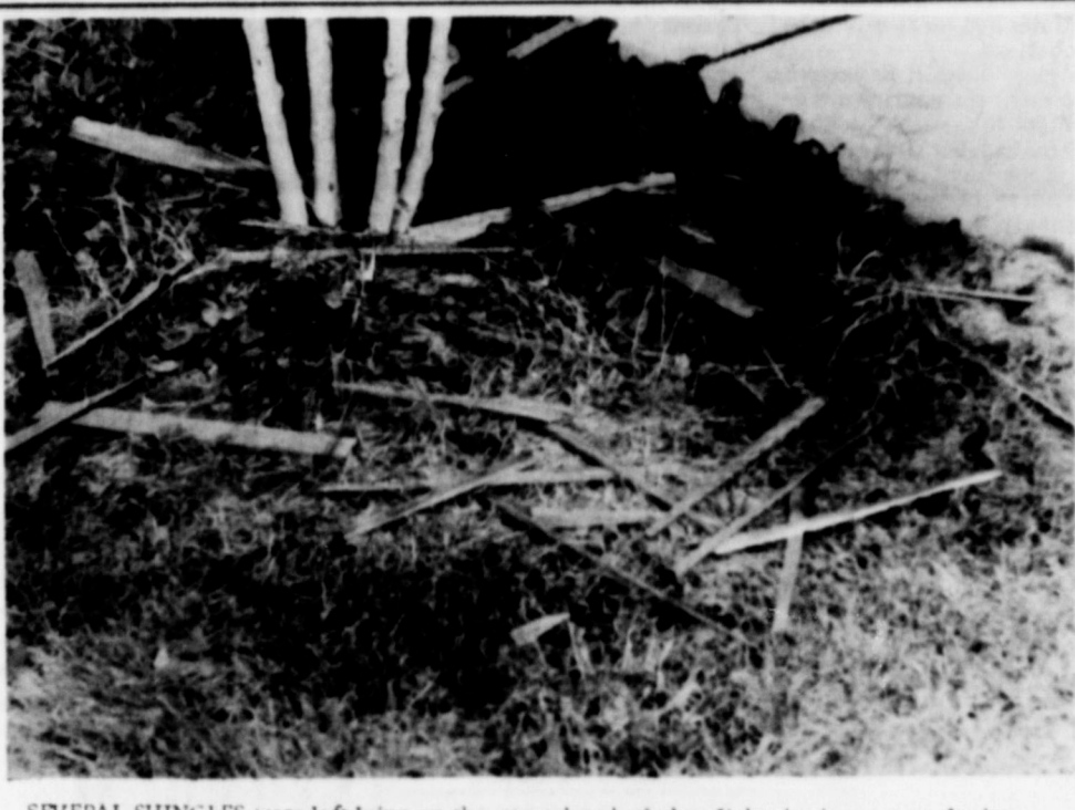
SEVERAL SHINGLES were left lying on the ground and window lights broken out at the home of Representative Billy Wayne Clayton, following the hail storm Saturday.
