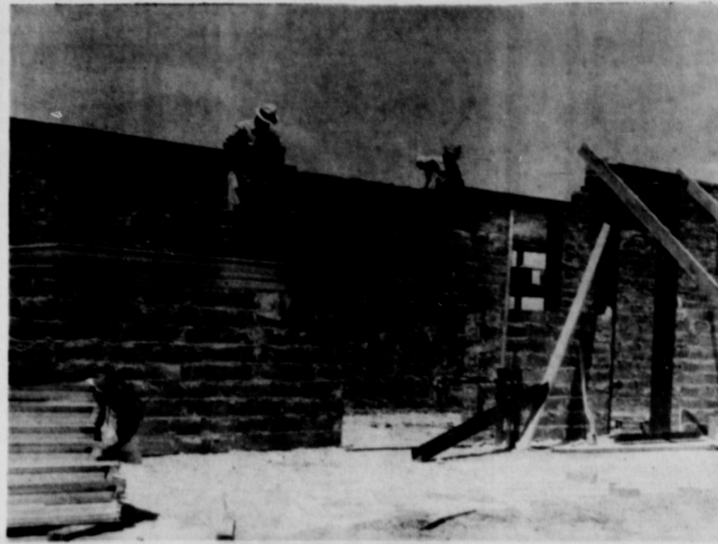
UP GO THE WALLS.. of the addition to the Springlake Elementary Building, which will include a new library, very much needed by Elementary students. The new class rooms being added will ease the crowded conditions now existing.
