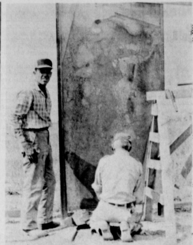
FARM CHEMICAL BUILDS ADDITIONAL FACILITIES--The initial phase of installing steel panels has begun at the Farm Chemical Co. The new structure, 54' x 26' will be constructed of 12 gauge steel, and is due to be completed within the next few weeks. It will contain a partitioned office section and storage for different analyses of bulk fertilizer. Shown here are Norman Hinchliffe and George Miller.
