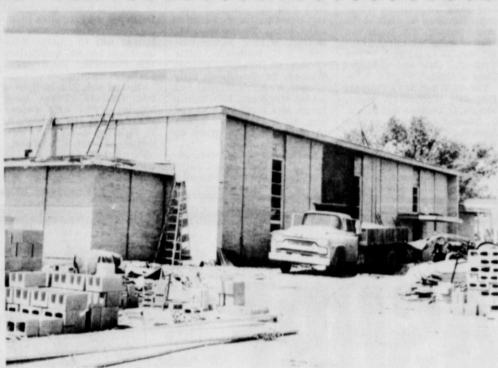
STUDENTS WILL BE EATING IN STYLE when the new Springlake School Cafeteria is completed. Every day, notable progress on various building projects is easily observed. All buildings under construction are progressing on schedule, and the cafeteria is scheduled to be completed around October 1.
