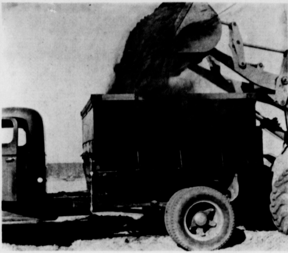
FROM HERE TO THERE... This rich (Earth near Earth) located at Springlake School is being moved from the track ground to be used later in connection with the construction of the new cafeteria.
