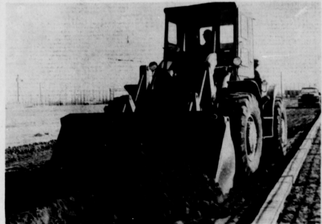
FILL IT UP TO THE BRIM... Workmen started this week getting the top surface removed from the Springlake track in preparation for a new face.
