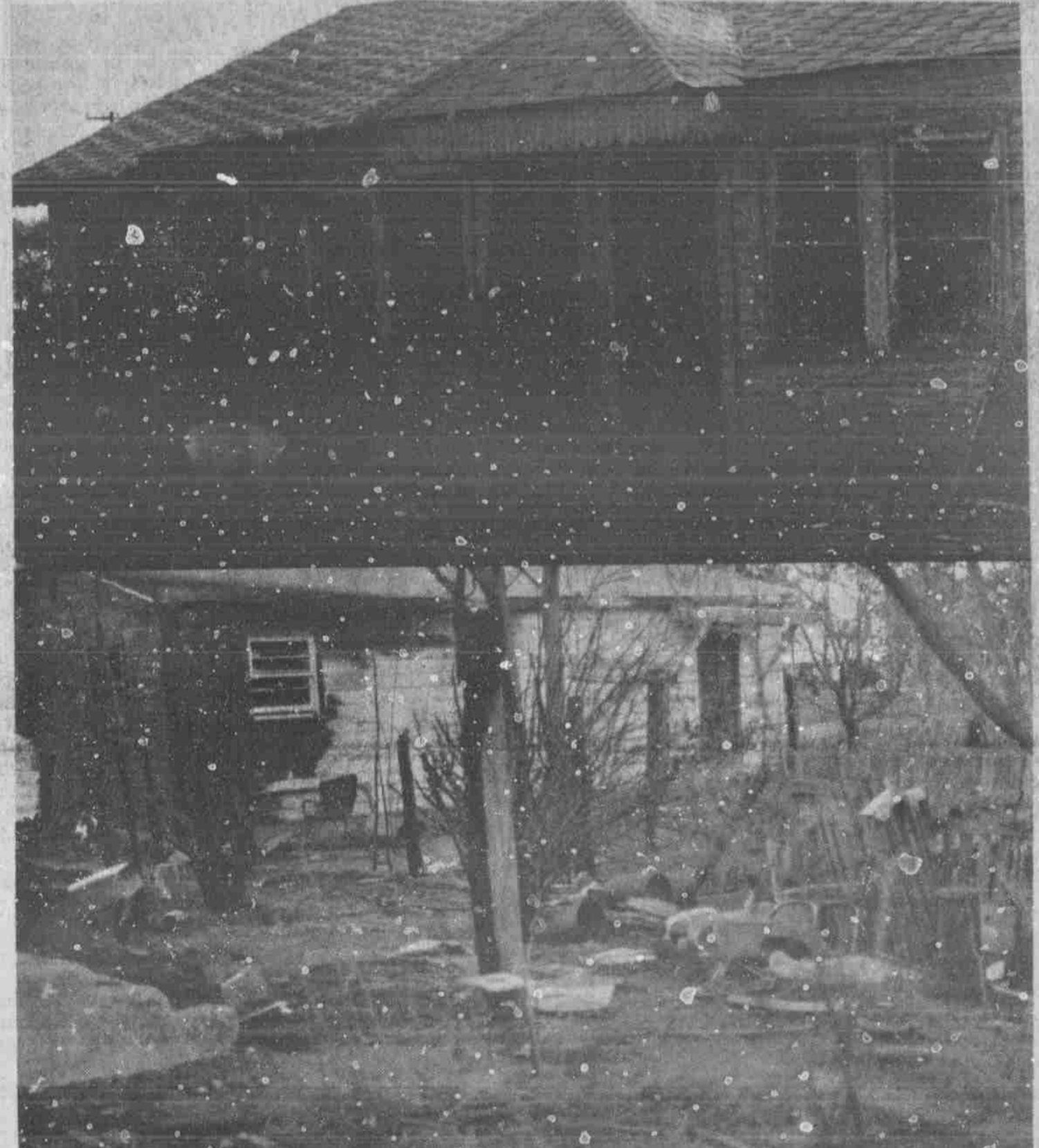
There is no doubt about it, something should be done about this situation which exists in "East Lubbock". The top photo is what was once a livable dwelling in the 1800 block of Avenue B. No one resides in this house, but it still stands. Why? The bottom photo is a scene of a recent house which was destroyed by fire several weeks ago. This house is located in the 2200 block of Cedar Avenue. Perhaps City Officials will pay attention to these "blighted areas in the Black community." (Staff Photo)
