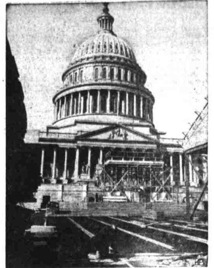
PREPARING FOR BIG DAY —Inaugural stand rises at Capitol, Washington, as preparations get under way for inauguration of Dwight D. Eisenhower as President, January 20.
