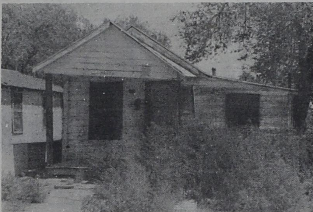
Tagged as substandard housing, this structure will be demolished by the city if the owner does not repair the housing to minimum standards.
