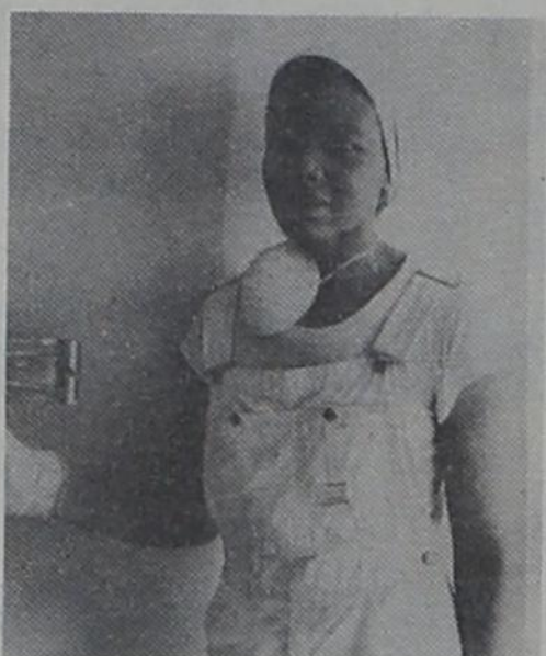
Rise Edgenton sands newly taped wall as part of her duties as an apprentice drywall taper.
