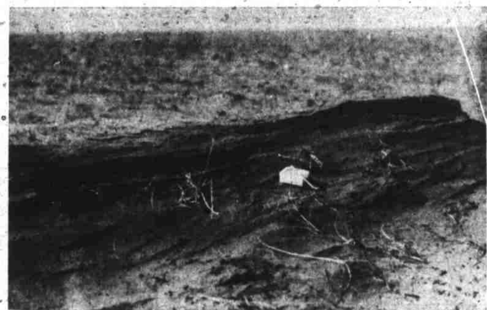
Example Of Severe Erosion
