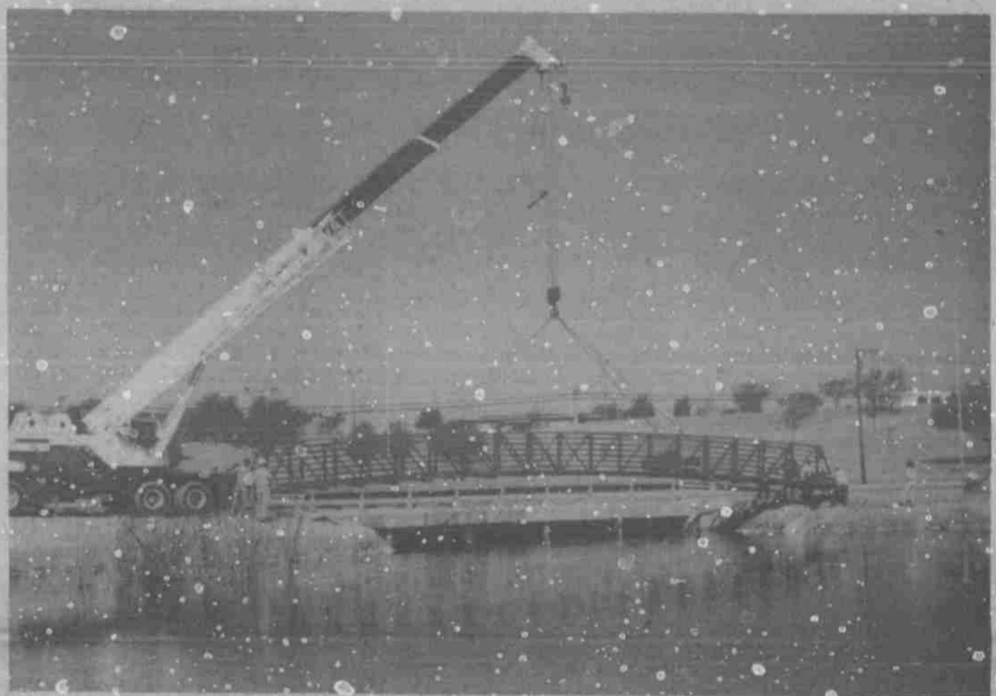
Here it is ladies! Pictured above is the construction of the Martin Luther King, Jr. Blvd. bridge which is in its final stages of construction as of this week. This photo was taken last Thursday afternoon. The project was constructed as a pedestrian foot bridge across Canyon Lake Six at MLK Blvd. The bridge will be located on the east side of MLK Blvd. to facilitate pedestrians crossing along MLK Blvd. without walking on the roadway.
