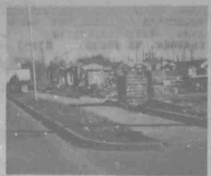
BLACK LUBBOCK GONE!! The demolition of Black Lubbock. The "Flats" as it has been called for many years is the last of the original Black community. This destruction is making way for the new Interstate 27.
