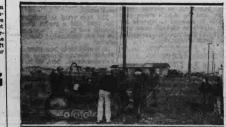
Pole Holes Frosts—Power for locomotion and for boring holes almost on the run. This modern power line crew is made up of E. E. Dozier, left, and J. P. Gilmer, both of Fort Worth, and two helpers. New construction or reconstruction is their "meat."
