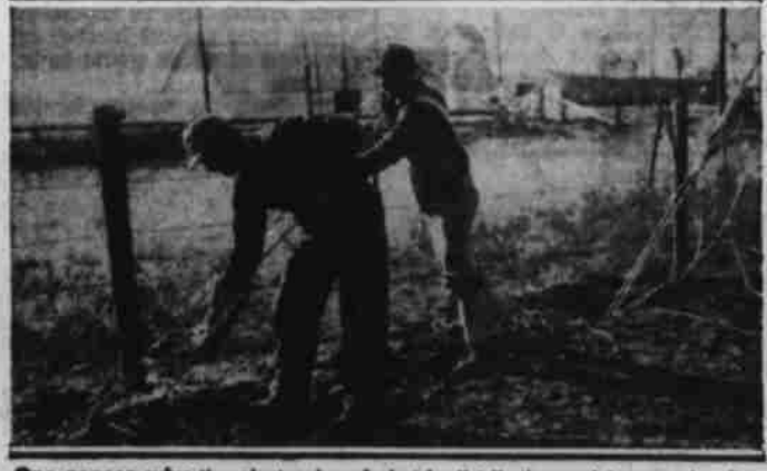
One reason why the giant poles of electric distribution and transmission lines can withstand the terrific strains that they do is because they are securely guyed wherever possible. Here Hazel Waddins and Wayne Gregston of Midland make secure the guy wires on a transmission line dead-end.
