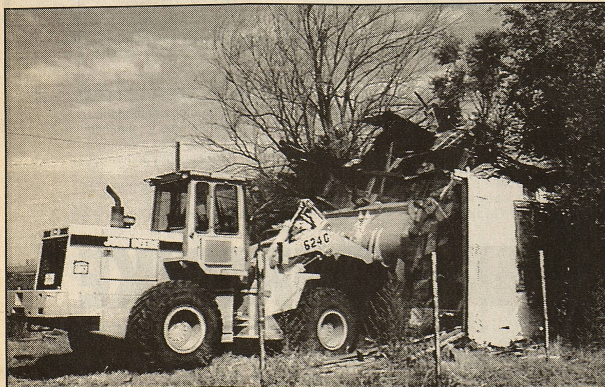
Pct. 4 employee Hershel Smith uses front end loader to crush house at 405 8th Street.
