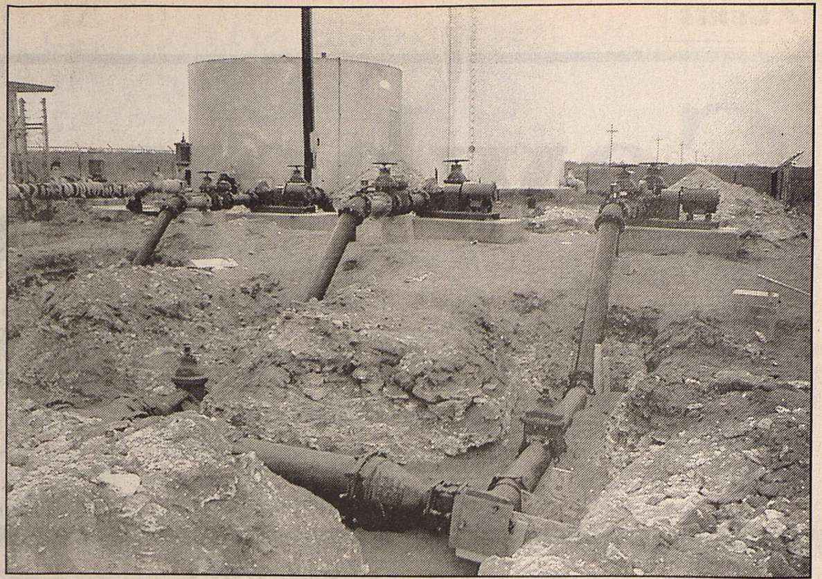
Work is nearing completion on the installation of a new water pumping station at the City's main storage tank southwest of town. City Administrator Ed Hansen said the old pumps were too ancient to be relied on, and when the new station is in operation the old equipment will be sold. The water passing through this pump station goes directly to the City's watertower on 16th street, and then into the city distribution system.
