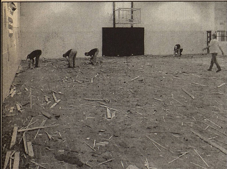
Workers are shown ripping up one layer of the floor of the Middle School Gym. The floor will be removed, "all the way to bedrock," a worker quipped.
