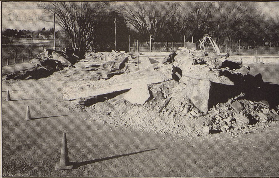
This pile of rubble was all that remained after County Precinct 3 personnel demolished the old bath house at the county pool in Stanford Park. West Texas Concrete submitted the low bid to construct a new, 1200 square foot building, and work should start on the project in the next few days.
