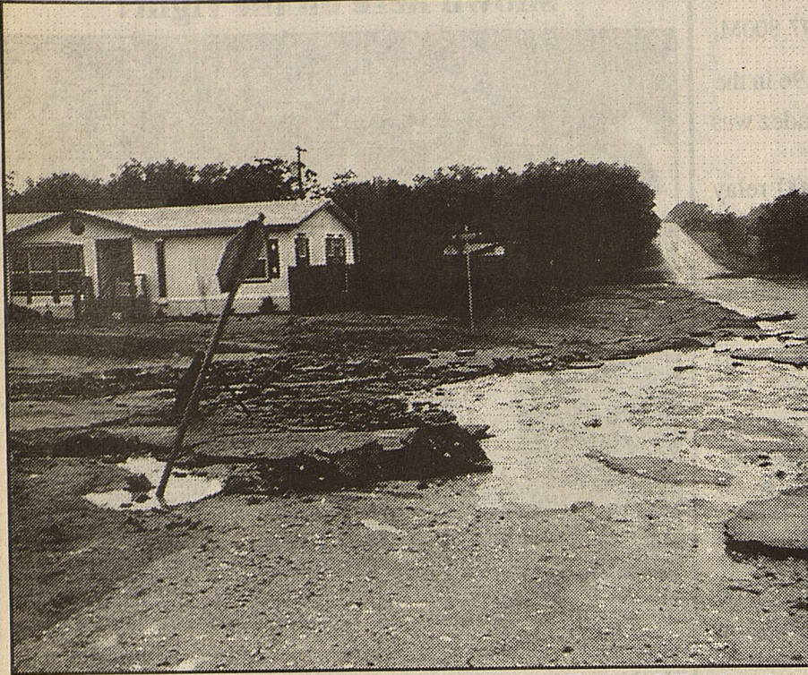
Several streets around town were damaged by runoff water following the rain front of the Jack Lowe residence.
