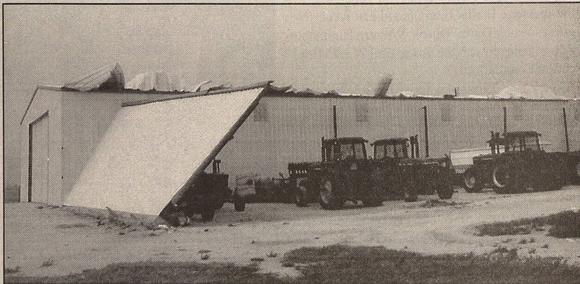
Tractors and equipment shown were completely covered by a pole barn structure the length of the main enclosed barn, before estimated 60 to 70 miles per hour ripped the structure away.
