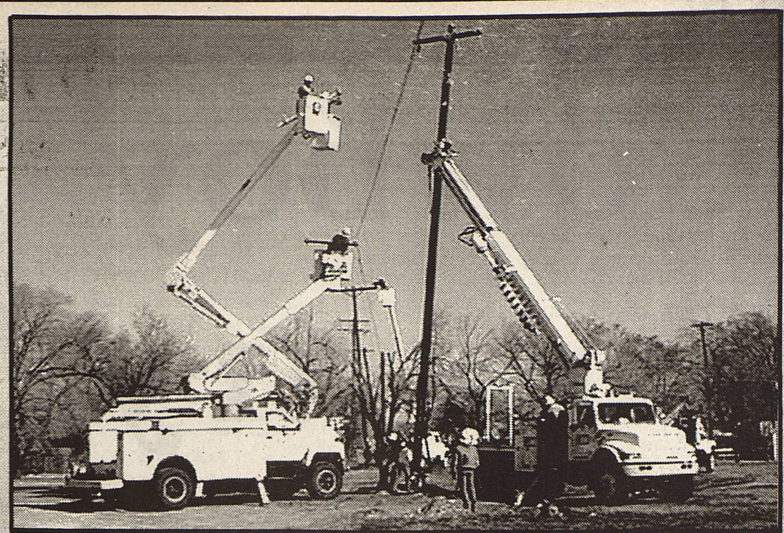
Lea County Electric Crews have now completed approximately 2/3 of the line conversion within the City of Plains. The projected completion date for all work is July, 1999. In this photo, Lea County Electric linemen work to replace a pole while keeping the line energized. Precision maneuvers like this are all in a day's work for the power professionals.
