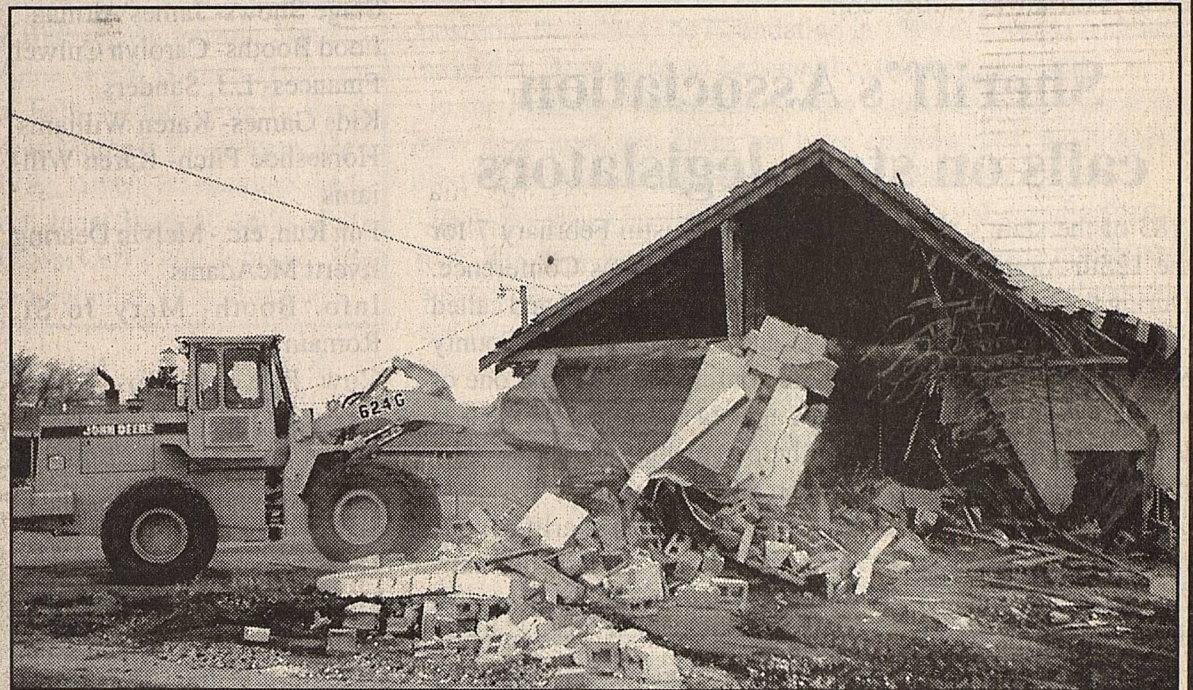
Precinct 3 employees made short work of demolishing the old Art Association building, completing the project in one day last Wednesday. All of the material was hauled to the county landfill. Hershel Smith is shown operating the loader used to demolish the structure.
