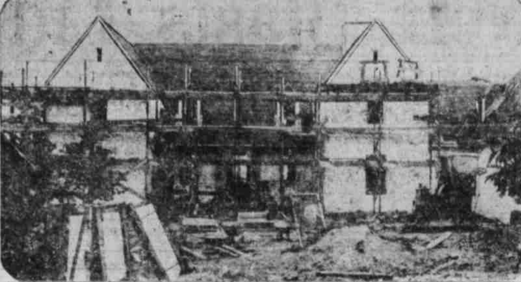
The above picture shows the progress made on the new home of Colonel and Mrs. Charles A. Lindbergh which is situated on Bourland mountain six miles from Princeton, N. J.
