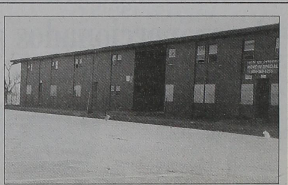
This week, Judge Doty issued a 30 day order for demolish on the Villa Del Norte apartments, 1913 Baylor. That means the owner has 30 days to bring the apartment complex up to code. If the owner does not accomplish that within the 30 day period, the City can take further action against the owner including, but not limited to, demolishing the apartment complex.
