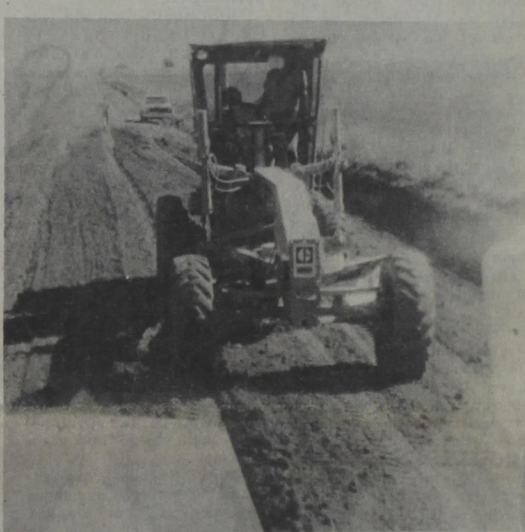
Commissioner Solis—Driving a caterpillar grader is not an easy job. Solis is seen here on the job, with fellow worker, "Skeet."
