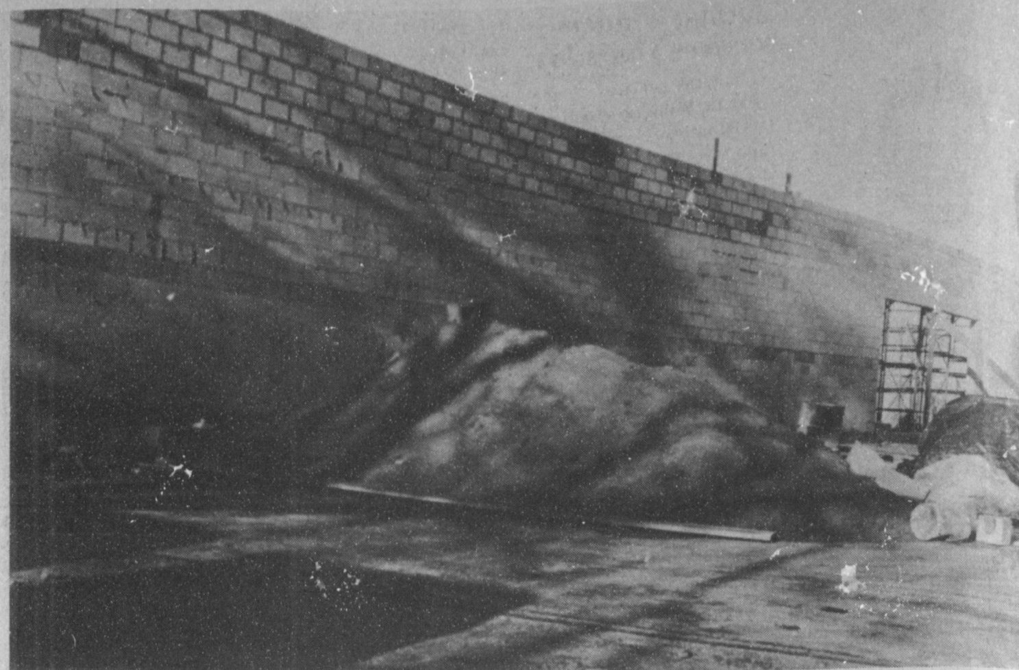
PAY AND SAVE CONSTRUCTION CONTINUING-- Walls are going up at Pay and Save Grocery at West Sixth Street and American Blvd. in the local grocery store's renovation and enlargement project. The size is being increased on the north side, and the entrance to the store has been moved to the west side of the store.
