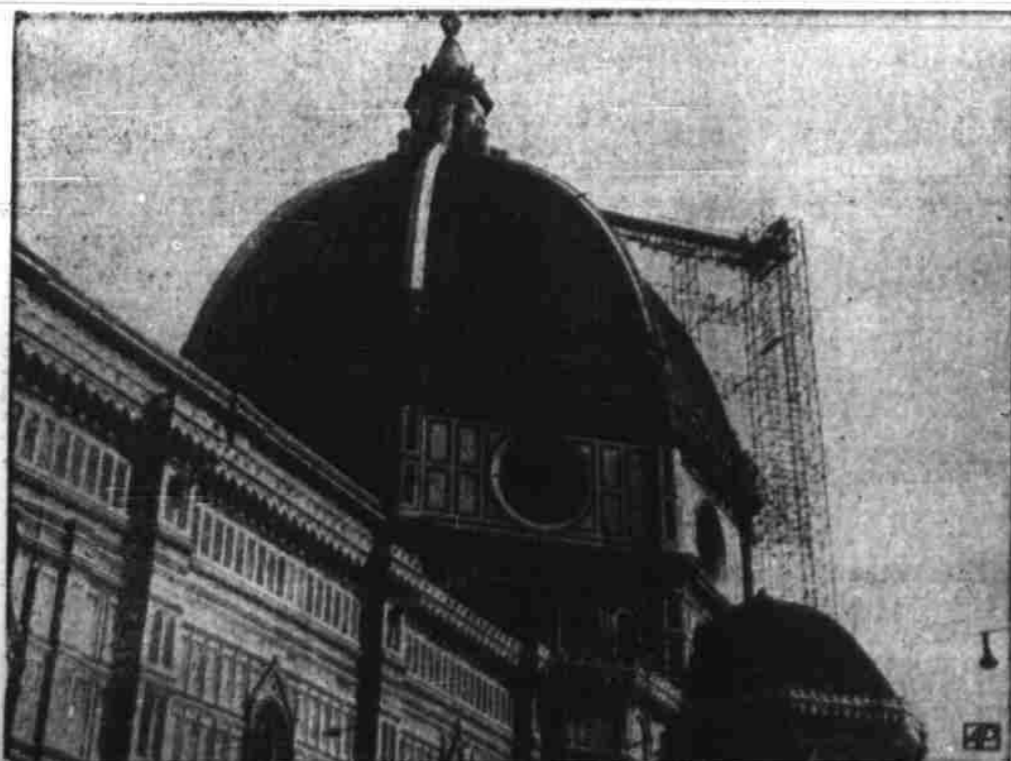
THE DUOMO GETS SHAMPOOED — The Duomo, Santa Maria del Fiore, world-famous Florentine church designed by Arnolfo di Cambio in the 13th century, is covered with scaffolding as workmen give its tiled roof a general overhauling to remove ravages of time.
