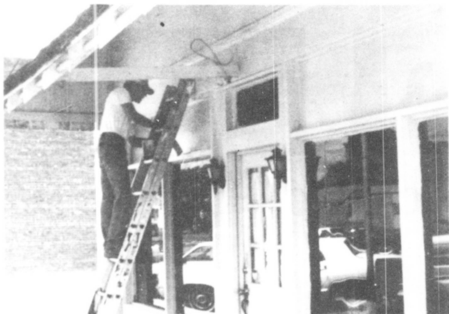
Jim Ridgeway paints the McAnear Insurance building in preparation of the Rodeo coming up this weekend. The Route 66 Mural will be hung on the south side of the building.
