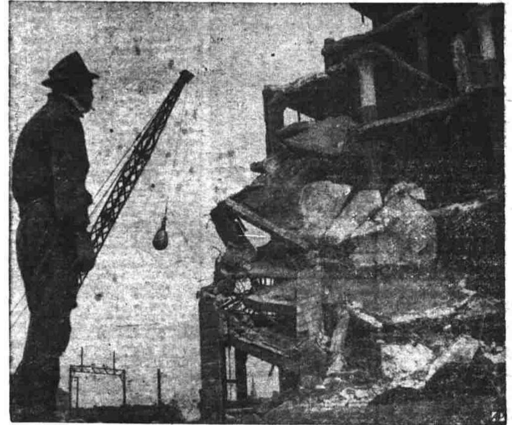
LOOK OUT BELOW! —An eight-story concrete building comes tumbling down in Philadelphia under the heavy blows of a swinging steel ball. Engineers used the ball, hung from a 70-foot crane boom and swung like a clock's pendulum, to raze the building for a new housing project. In this "angle" shot, a workman watches results.
