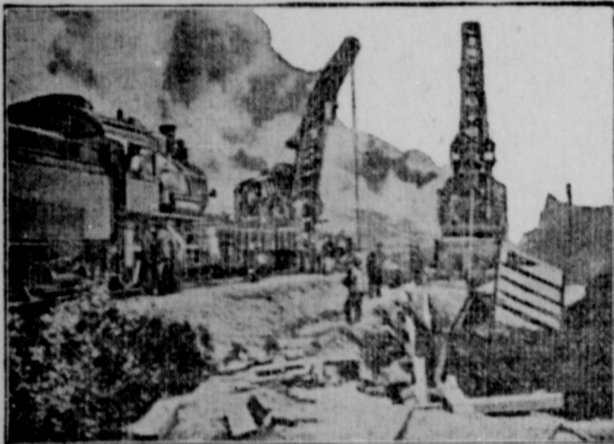
Drawing One of Three Freight Cars Out of a Sink Hole Under the Roadbed of an Eastern Railroad.
