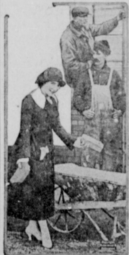
Mrs. Earl Carroll, wife of the Earl Carroll, the American composer, helping lay bricks for the flooring of her new bungalow on the roof of the Godfrey building at Seventh avenue and Forty-ninth street, New York. The bungalow will cost over $40,000, and it took Mr. Carroll three years to find a suitable place to erect his "suburban" home. Surrounding the bungalow, which is more than a bungalow, inasmuch as it will have eight rooms, will be in a fine Italian garden, with at least a five-foot brook crossed at intervals by stepping stones and rustic bridges. The ground about the villa will contain a vegetable garden, a handball court and an orchard consisting of two apple trees.
