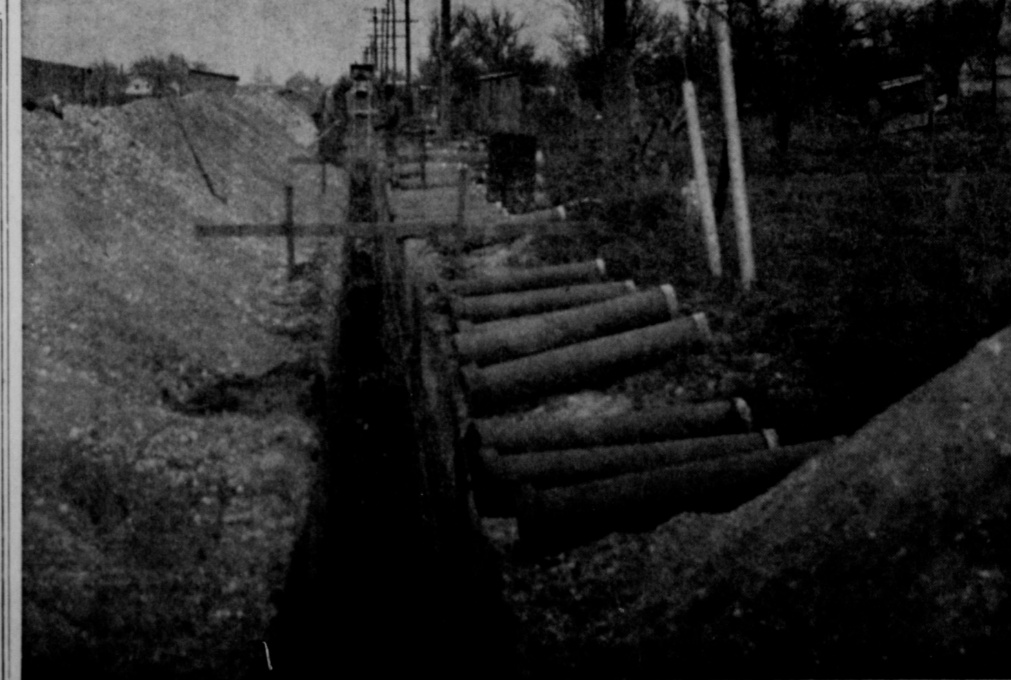
SLATON IS GROWING—Extension of sewer facilities in a town is one sure sign of its progress and growth. Construction of a new outfall line from the disposal plant, construction of a life station, and sewer mains
