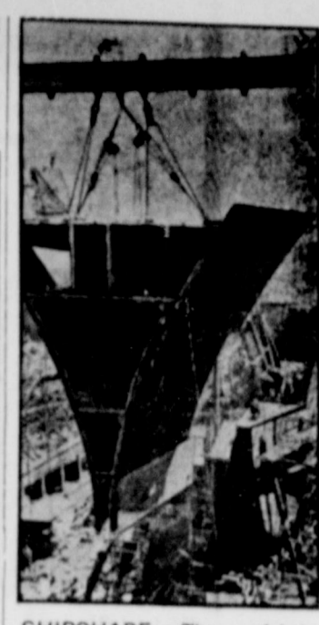
SHIPSHAPE — The prefabricated bow section of the S.S. Golden Mariner is seen above being lowered into place at San Francisco, Calif., shipyards. Once in position, it was shored up and welded to structure.
