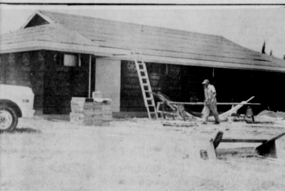
GOING UP — St. Thomas Clinic, being built for Dr. Ernesto Maldia, is scheduled to be completed by July 1, according to Ebb Stricklin, builder. The clinic is located at 22 and Knox Sts. and has been under construction less than a month. (SLATONITE PHOTO)
