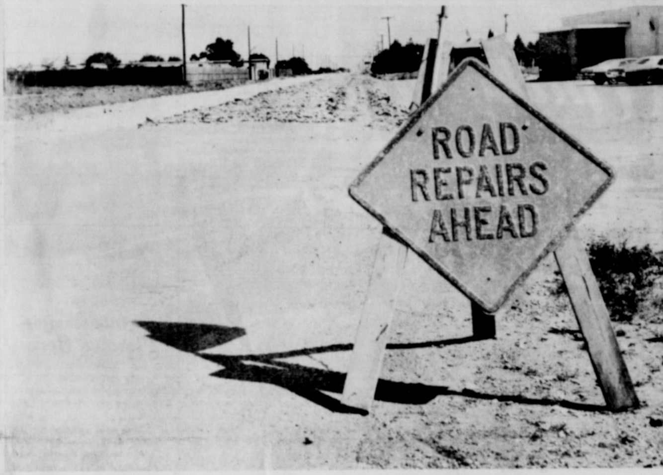
PAVING AT LAST — The 20th Street chughole trail at last is being resurfaced, with work getting underway this week along the portion leading up to Industrial Drive on the north end. (SLATONITE PHOTO)
