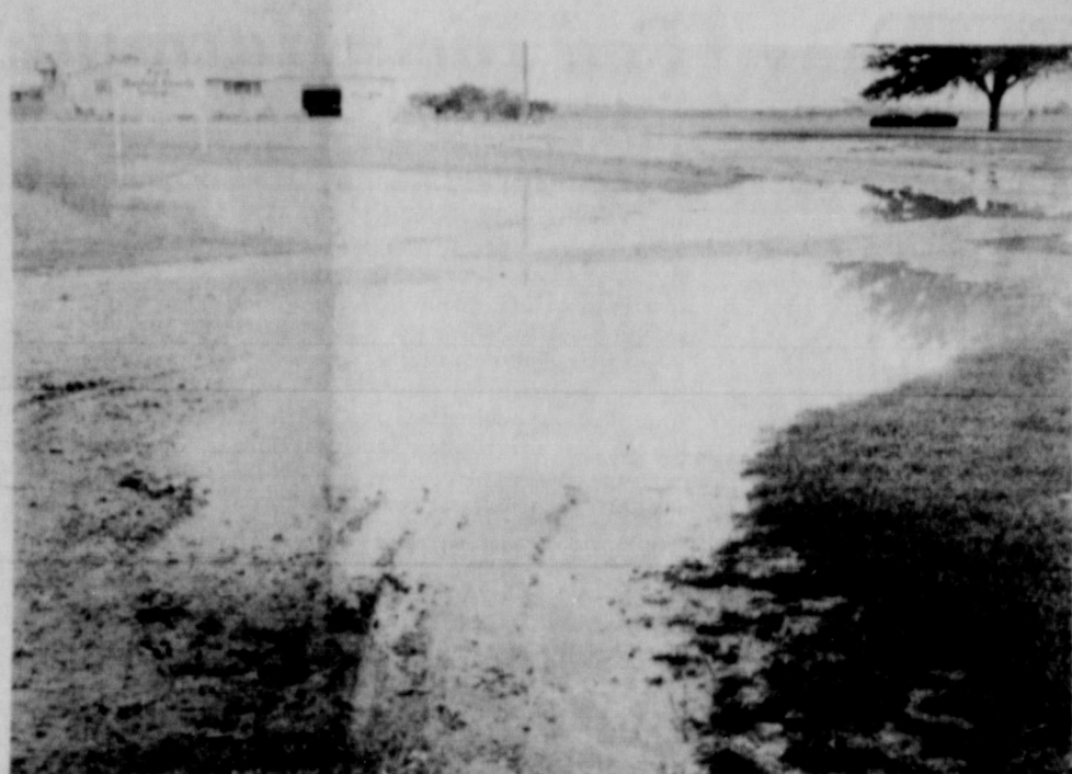
this not only inconveniences school children and churchgoers, but also residents of homes along the road. Now, the residents say, high water overflowing from the road has ruined two water wells of residents, and poses a threat to the drinking water wells for the church, school and clubhouse. (SLATONITE PHOTOS)
