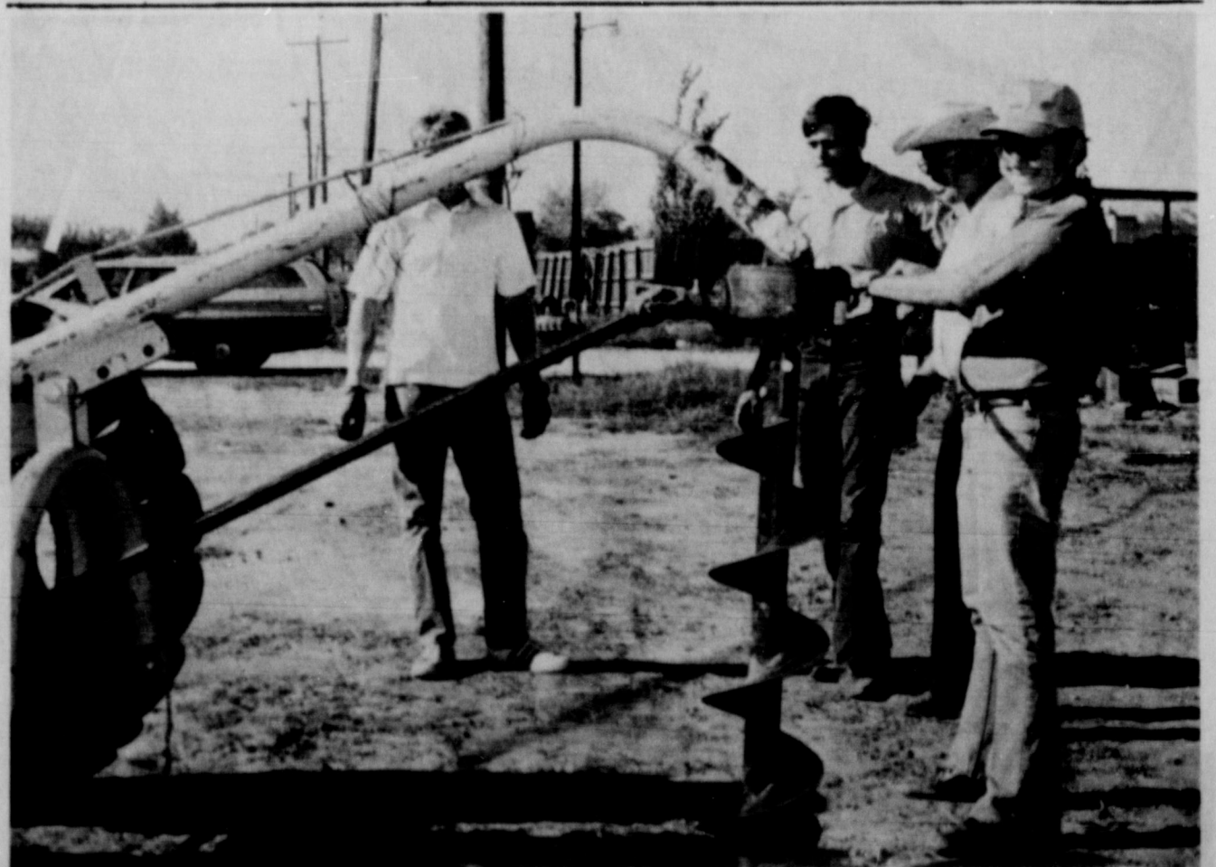
JAYCEES ON PLAYGROUND —These Slaton Jaycees were busy installing playground equipment at Stephen F. Austin School last Saturday. President Jim Dulin, operating the tractor, is not shown. The others, from left, are Steve Tucker (with no face), Danny Smith, Marlin Payne and Ted Dawson. (SLATONITE PHOTO)
