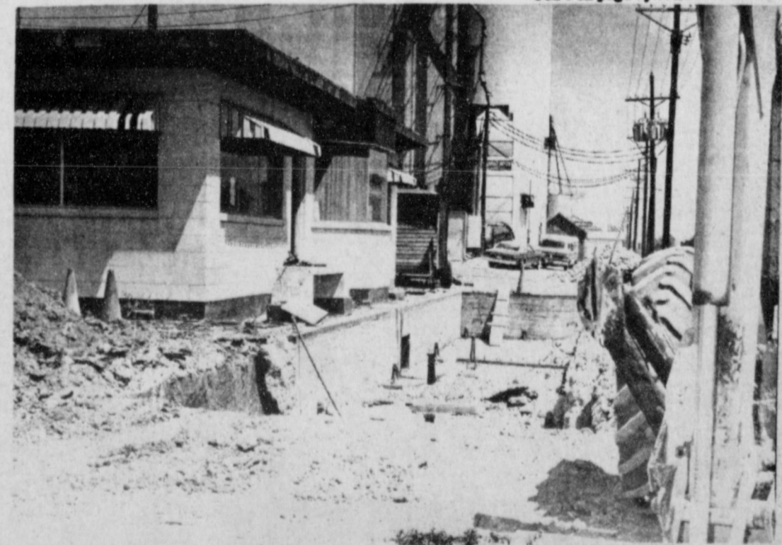
EXTENDING WEIGHT SCALES . . . Work has been under way for several days at Ray Griffiths and Sons Elevator removing existing scales and installing new scales which are longer enabling the elevator to weigh trucks with a larger load capacity. The increased size of Transcontinental shipping trucks has made the extension necessary.
