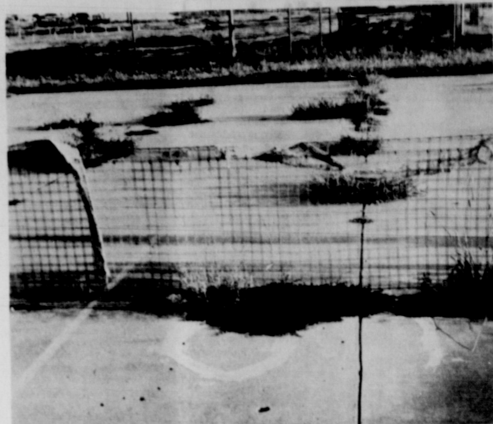
SLATON'S GRASS COURTS -- Two of Slaton's four tennis courts look like this, with grass clumps growing in the cracks on the playing surface, and dilapidated wire nets complementing the sagging backstops. (SLATONITE PHOTO)
