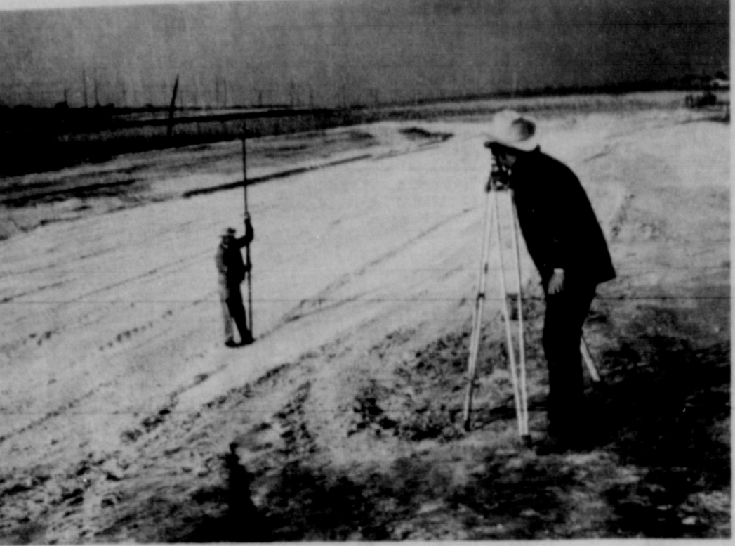
POLLUTION CONTROL PIT -- Engineering assistance is being furnished by the Soil Conservation Service through the Lubbock County Soil and Water Conservation District in the construction of pollution control pit on the Lubbock Christian College Feedlot north of Lubbock. (USDA PHOTO)
